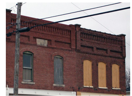
Examples of unrestored and boarded up windows
