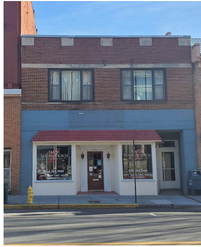
Example of inappropriate bulkheads and windows
