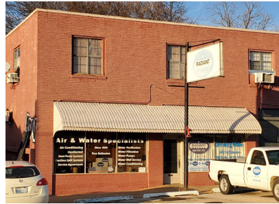
Inappropriate signage, lighting, and awnings
